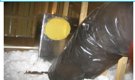
A disconnected return duct in the attic pulling unconditioned air and insulation into the furnace.
