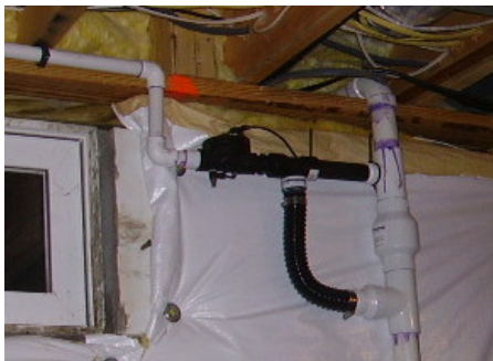
A typical water operated sump back-up that doesn't require electricity to run.
