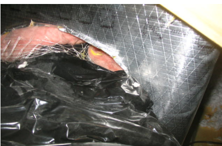
Open gaps in an attic supply duct.
