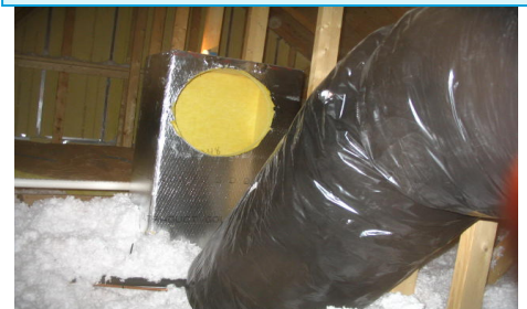
A disconnected return duct in the attic pulling unconditioned air and insulation into the furnace.
